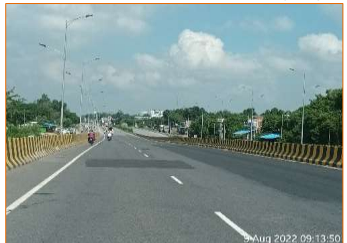
Pavement Condition at km. 779+600 (RHS)
