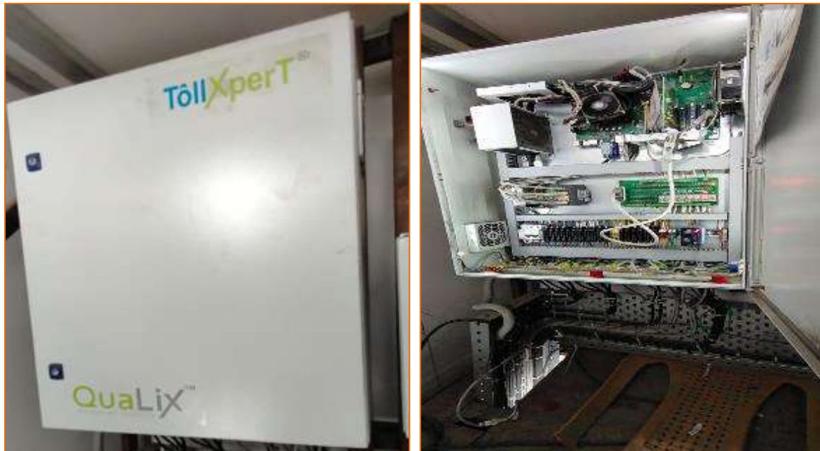
Figure 9-3 Toll Lane Controller TLC
