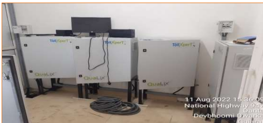
Figure 8-3 Lane Controllers for normal ETC lanes
