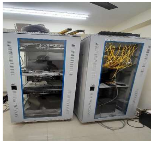
Figure 9-12 Control Room Equipment - Server & Switch rack
