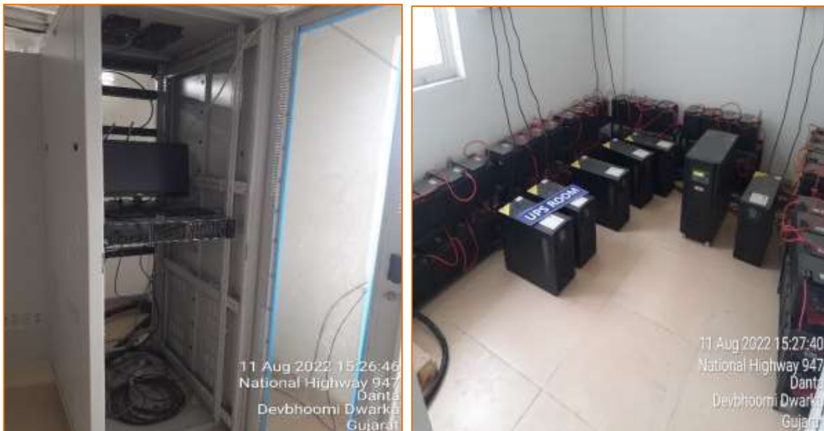
Figure 8-8 Control Room Equipment - Server & Switch rack/UPS Room
