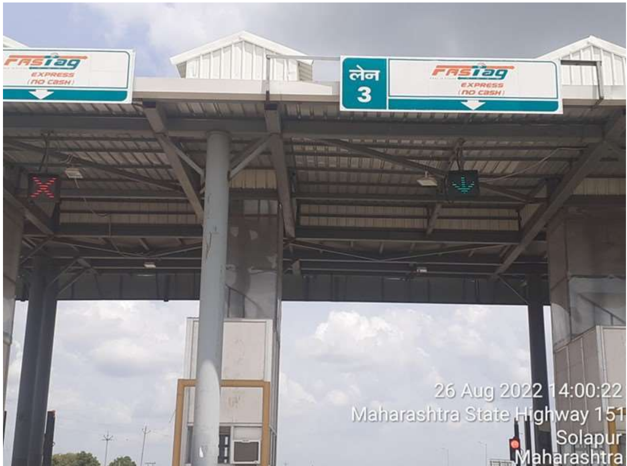
Figure 9-5 OHLS indicating green arrows for operational lanes
