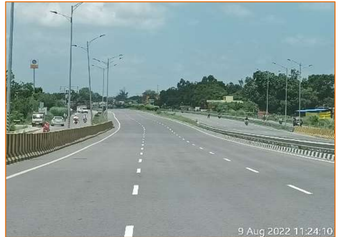
Pavement Condition at km. 722+100 (RHS)
