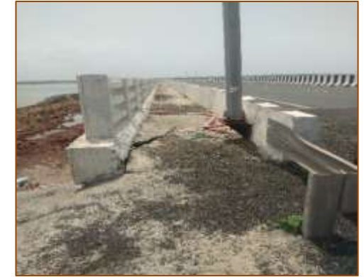
Major Bridge - km. 433+295 (RHS) Footpath settled
