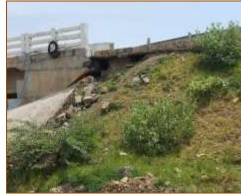
Settled CC Pitching at A2 side of MJB at km. 415+929 (RHS)
