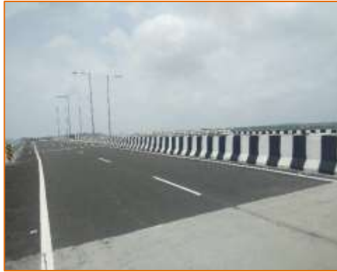
Wearing Coat of ROB at km. 0+527 (RHS)
