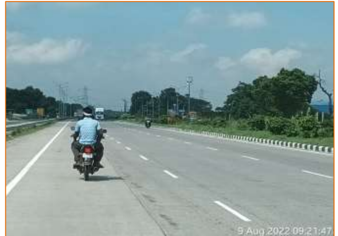
Pavement Condition at km. 785+650 (RHS)
