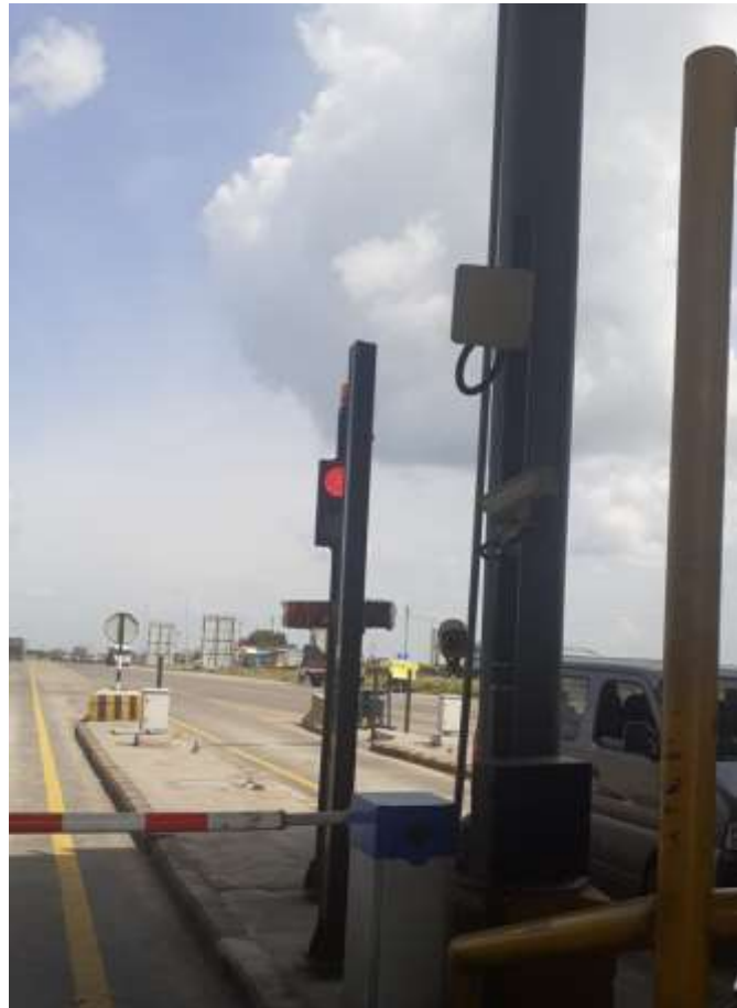
Figure 9-2 RFID ETC Reader mounted on Pole
