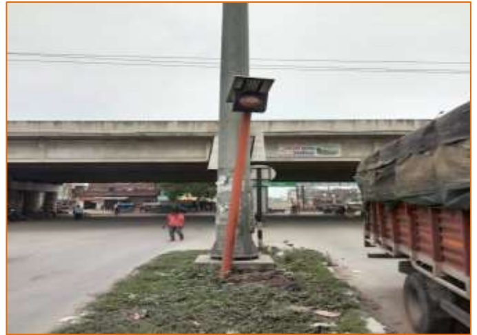
LED Blinker at km. 754+441
