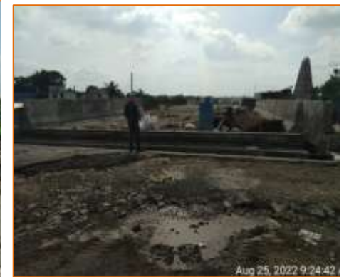
Expansion joint @ A2 side of Flyover is in progress at km. 136.857 (RHS)
