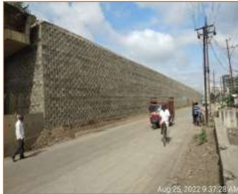
Friction slab & crash barrier of Flyover pending at km. 136.857 @ A2 side (RHS)
