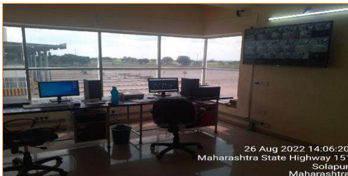
Figure 9-10 Incident Management Workstation at Control room
