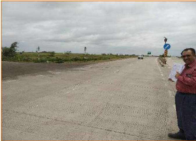
Pavement Condition at km. 306+500 (LHS)
