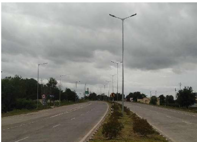
Highway Lighting at km. 313+700
