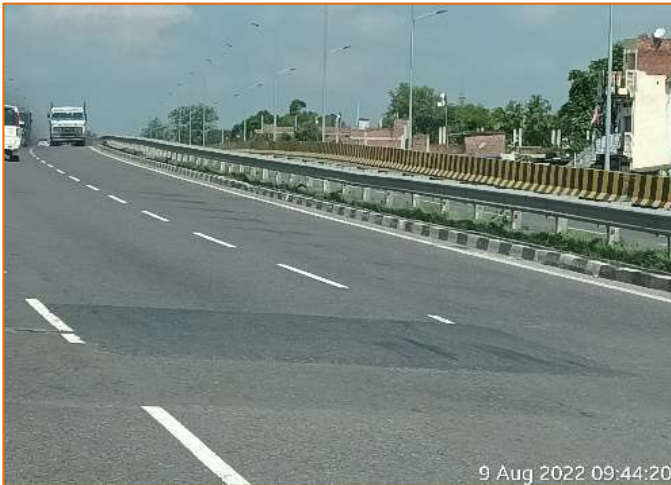
Pavement Condition at km. 765+100 (RHS)
