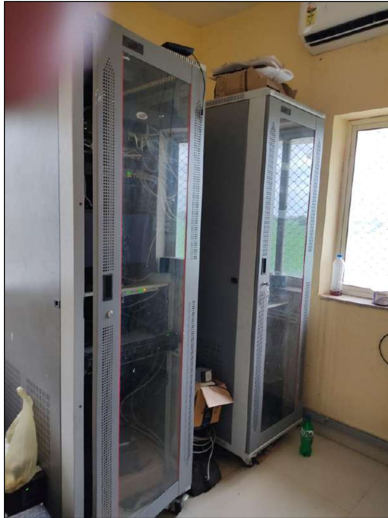
Figure 9-13 Control Room Equipment - Server & Switch rack
