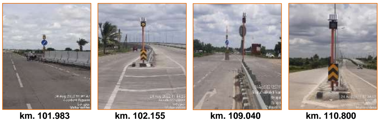
Figure 3-11 Photographs of Highway/Solar Lighting
