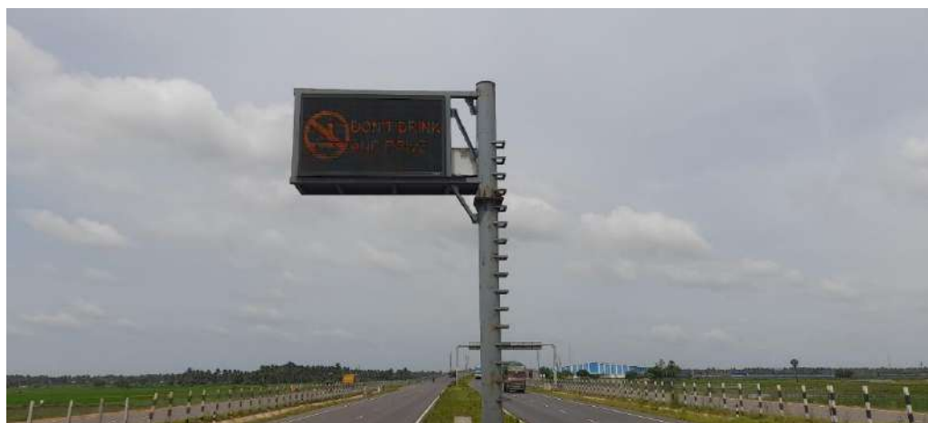
Figure 9-16 VMS on project highway
