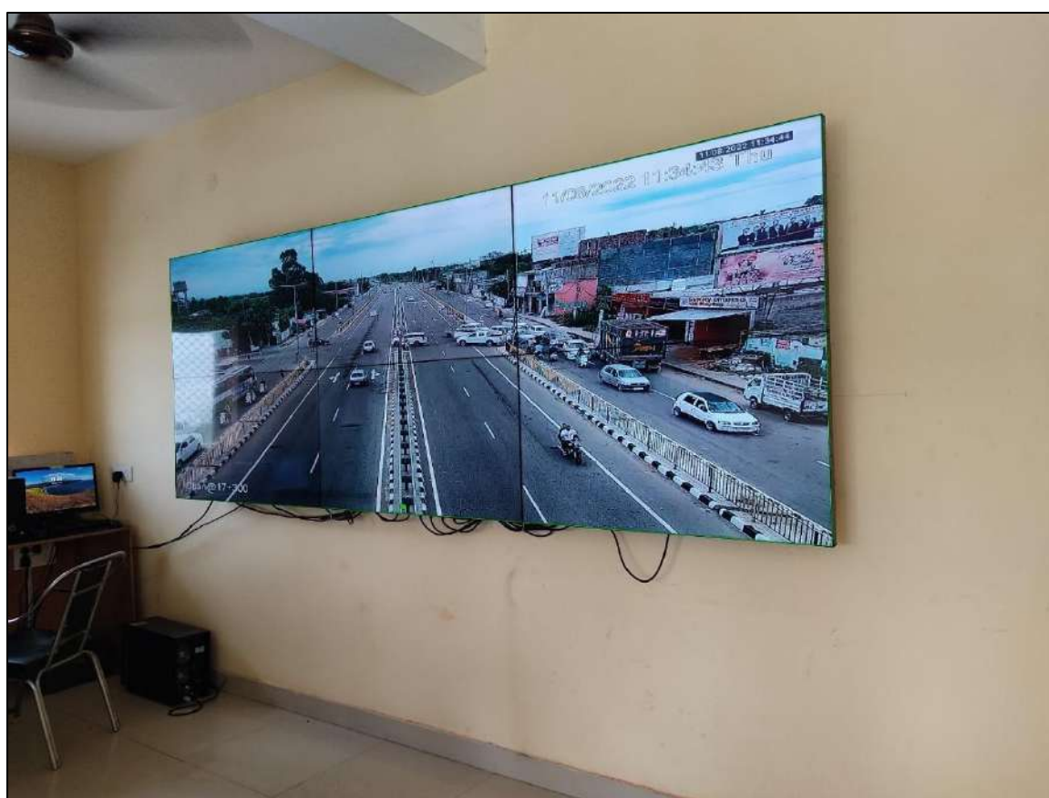
Figure 9-18 Video wall at HTMS Control room
