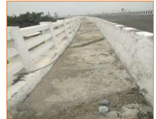
Uneven Drain with footpath at A1 side of MJB at km. 422.314 (LHS)
