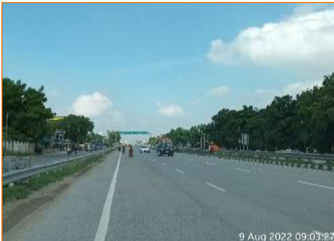
Pavement Condition at km. 785+200 (RHS)
