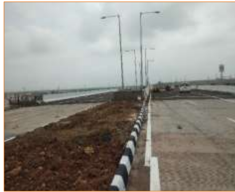
Wearing Coat of VUP at km. 12+420 (BHS)
