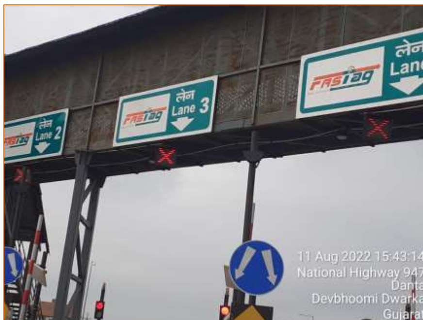
Figure 8-5 Over Head Lane Signal (OHLs)
