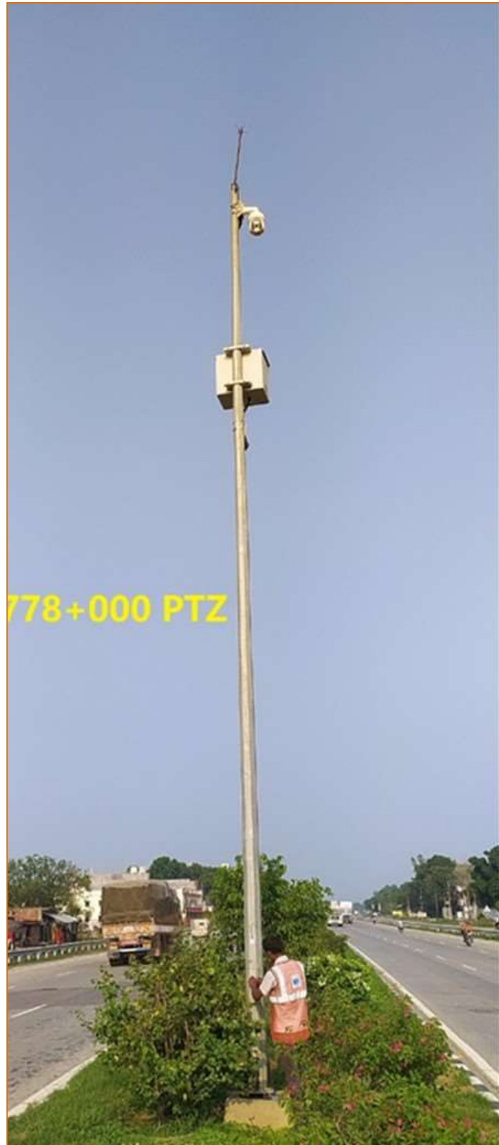
Figure 9-9 PTZ camera at km. 778.000
