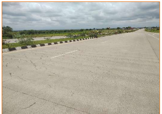
Pavement Condition at km. 304+600 (LHS)
