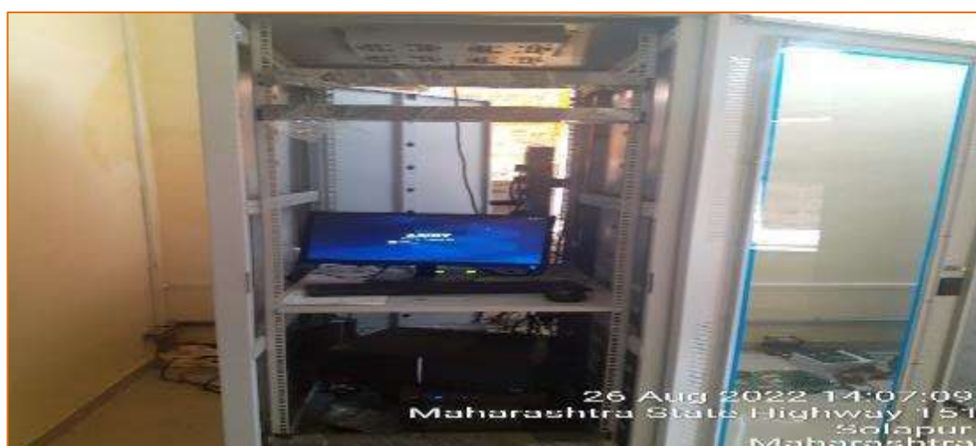
Figure 9-8 Medium Control Room Equipment – Server & Switch rack
