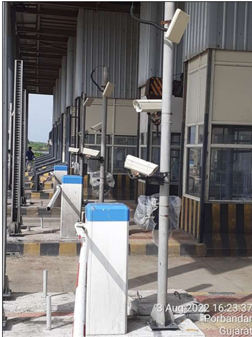
Figure 9-3 RFID ETC Reader mounted on Pole
