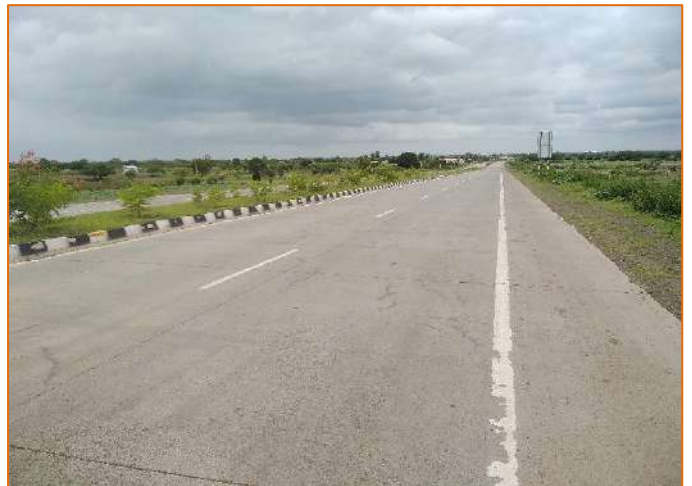
Pavement Condition at km. 319+100 (RHS)
