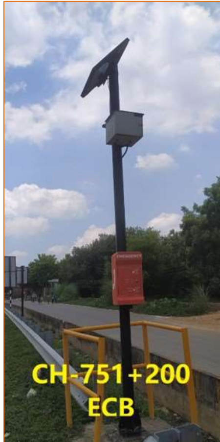
Figure 9-6 ECB at km. 751.200
