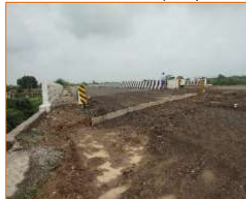
Wearing Coat pending of Major Bridge at km. 23+600 (LHS)
