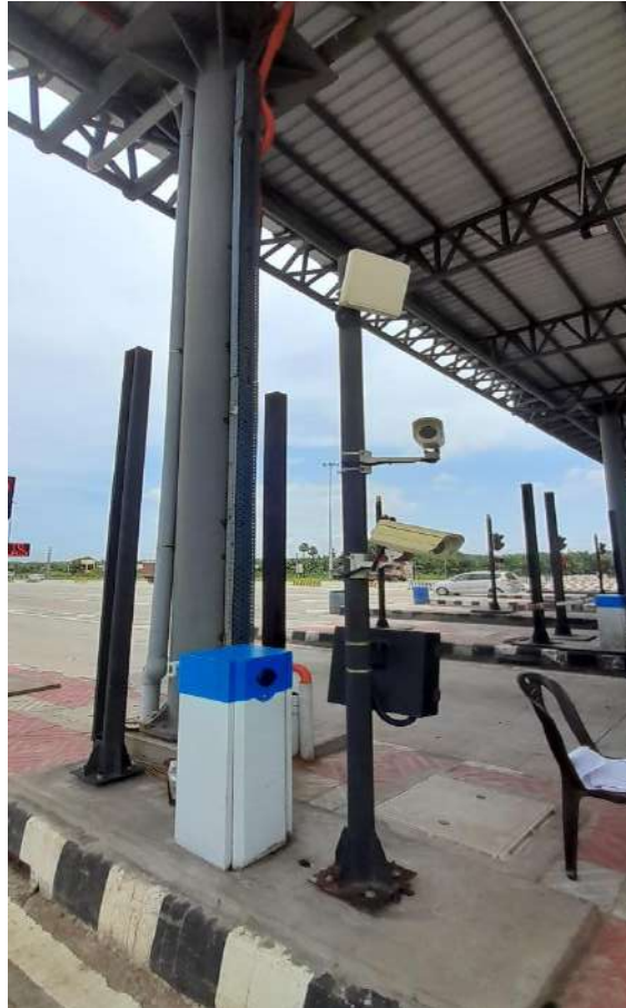
Figure 9-2 RFID ETC Transceiver installed on pole
