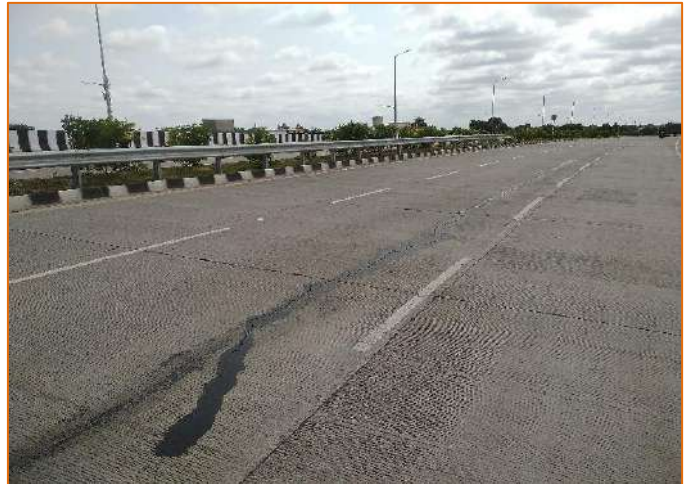
Pavement Condition at km. 287+700 (RHS)
