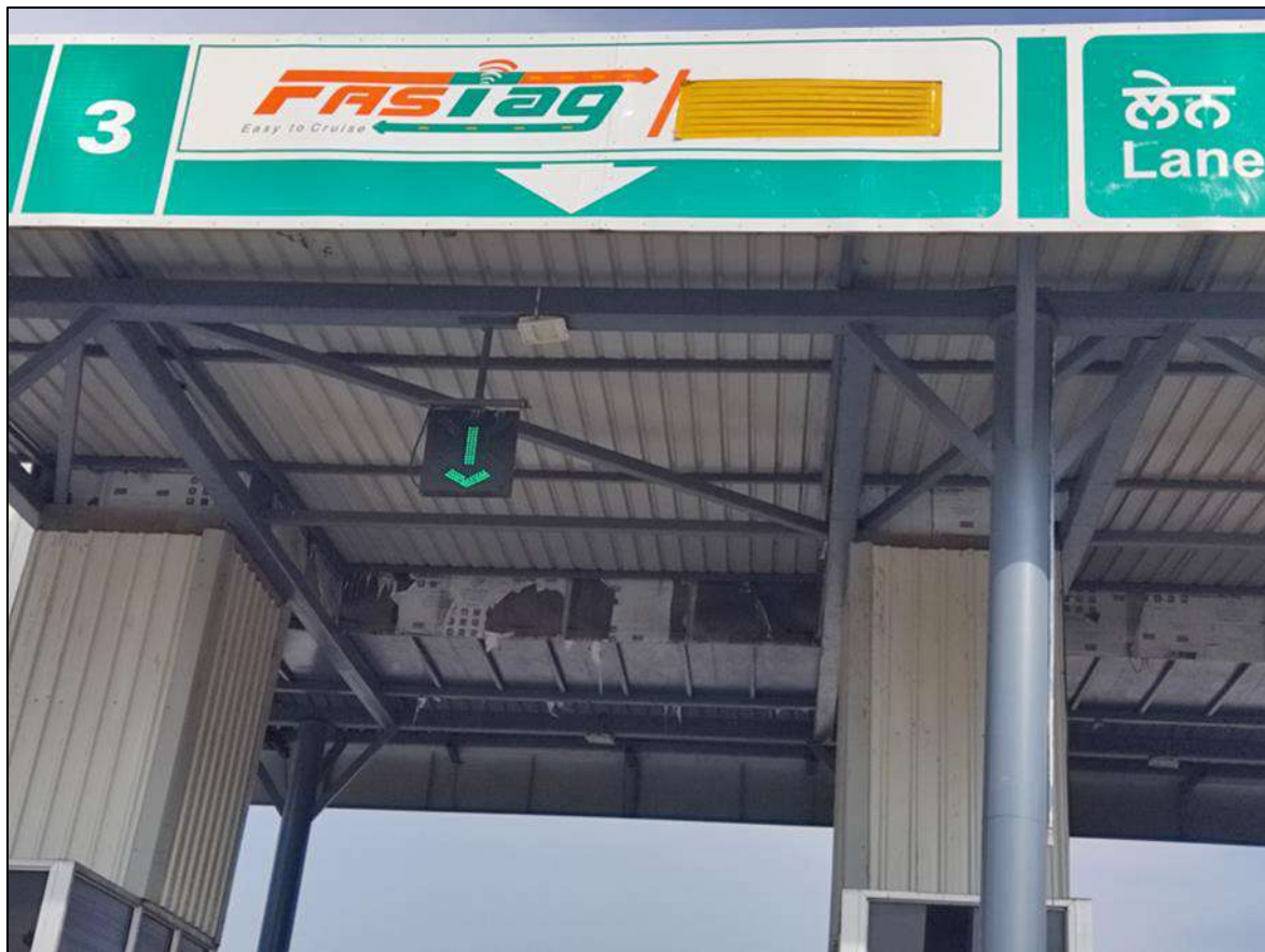
Figure 9-10 Over Head Lane Signal (OHLs)
