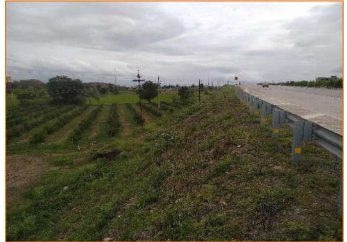
Crash Barrier at High Embankment Location
