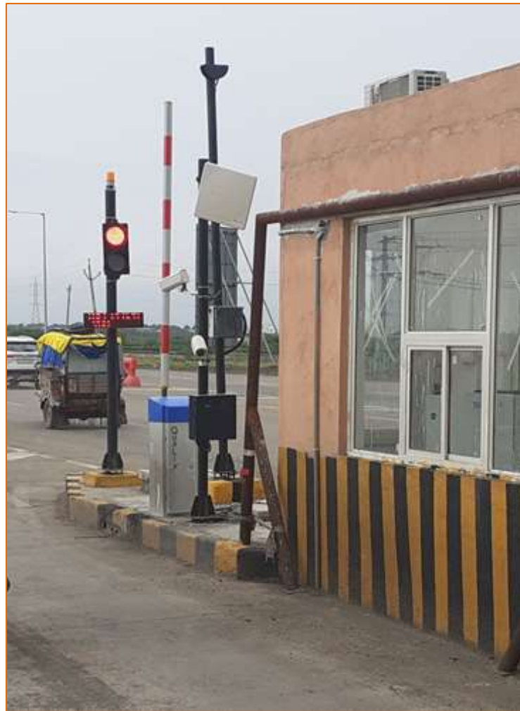
Figure 8-2 RFID Scanner located on pole
