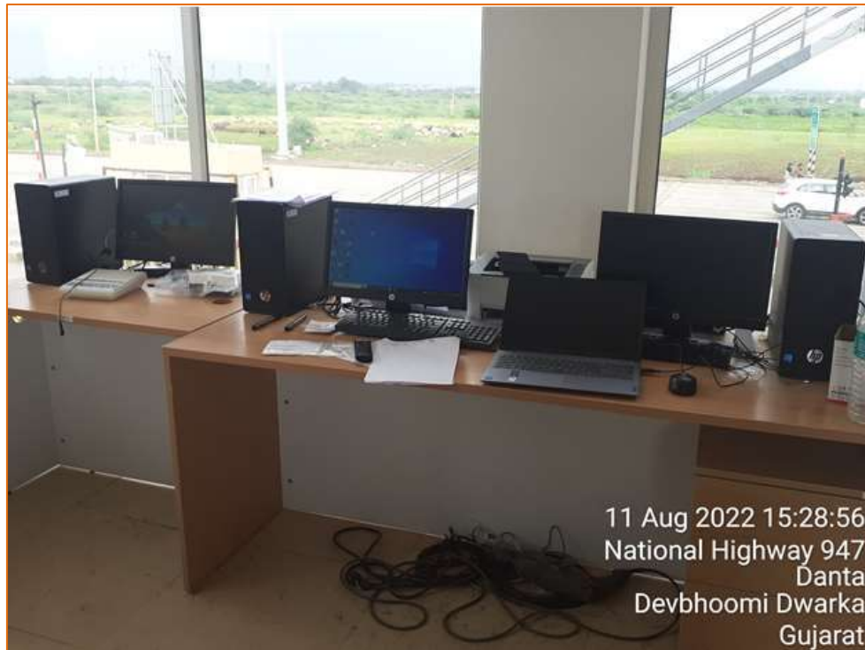
Figure 8-10 Workstations at Control room
