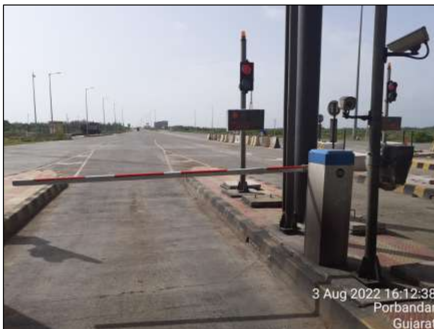
Figure 9-6 Automatic Lane Barrier
